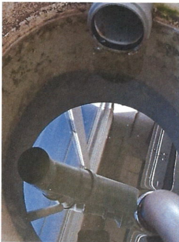
Picture 4 Treated water in inflow tank
